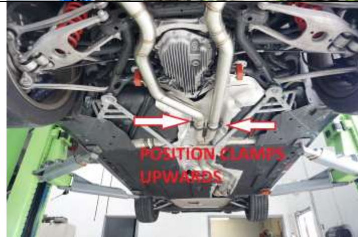
19. SNUG BALL CLAMPS (13MM) WITH BOLT END TOWARDS BOTTOM OF CAR. WILL NEED TO REPOSITION WHEN REAR EXHAUST ATTACHED.
